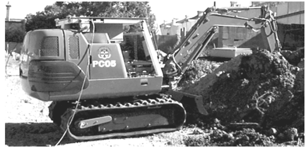
Fig. 1. Field machines such as the ACFR autonomous excavator pictured above are difficult to control directly at task-level due to dependency of the operational space controller on compensation of uncertain dynamics like compliance, friction and excavation reactions.
